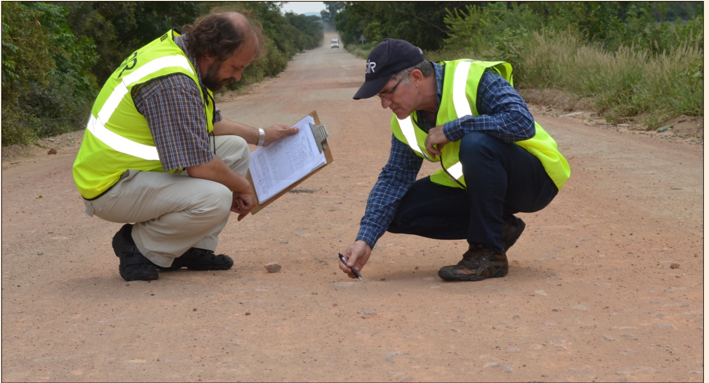
Louw du Plessis (right) and Dave Ventura (left) from Council for Scientific and Industrial Research (CSIR) during the visual inspection of Road D2808 from Sonop to Bokfontein. The 5,7km road is mostly used by the farming and mining communities in Brits and Sonop. A team of technicians and engineers from the CSIR's Built Environment unit is expected to go on a full scale soil sample collection at the road in two weeks.
